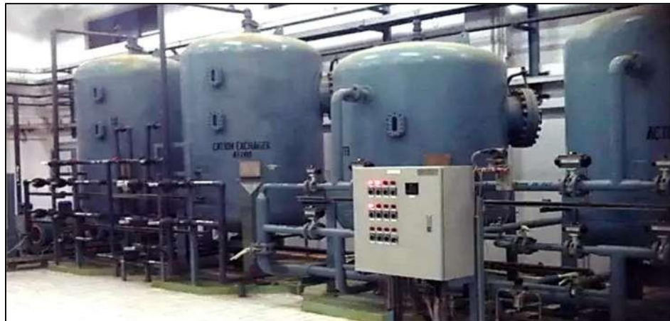
Fig.: Water DM Plant
